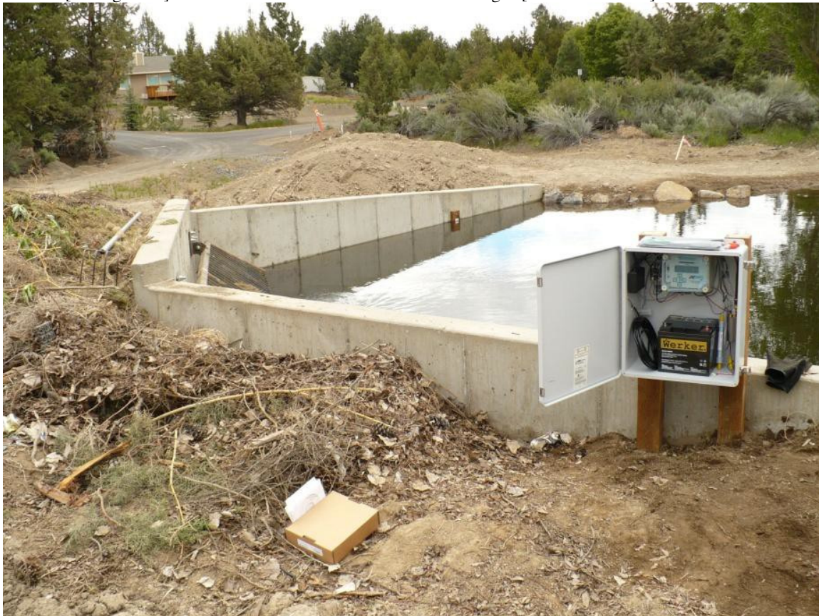
Figure 9. Measurement of water flow in an irrigation ditch, using the Stevens AxSys Flowmeter [Stevens Water 12].
